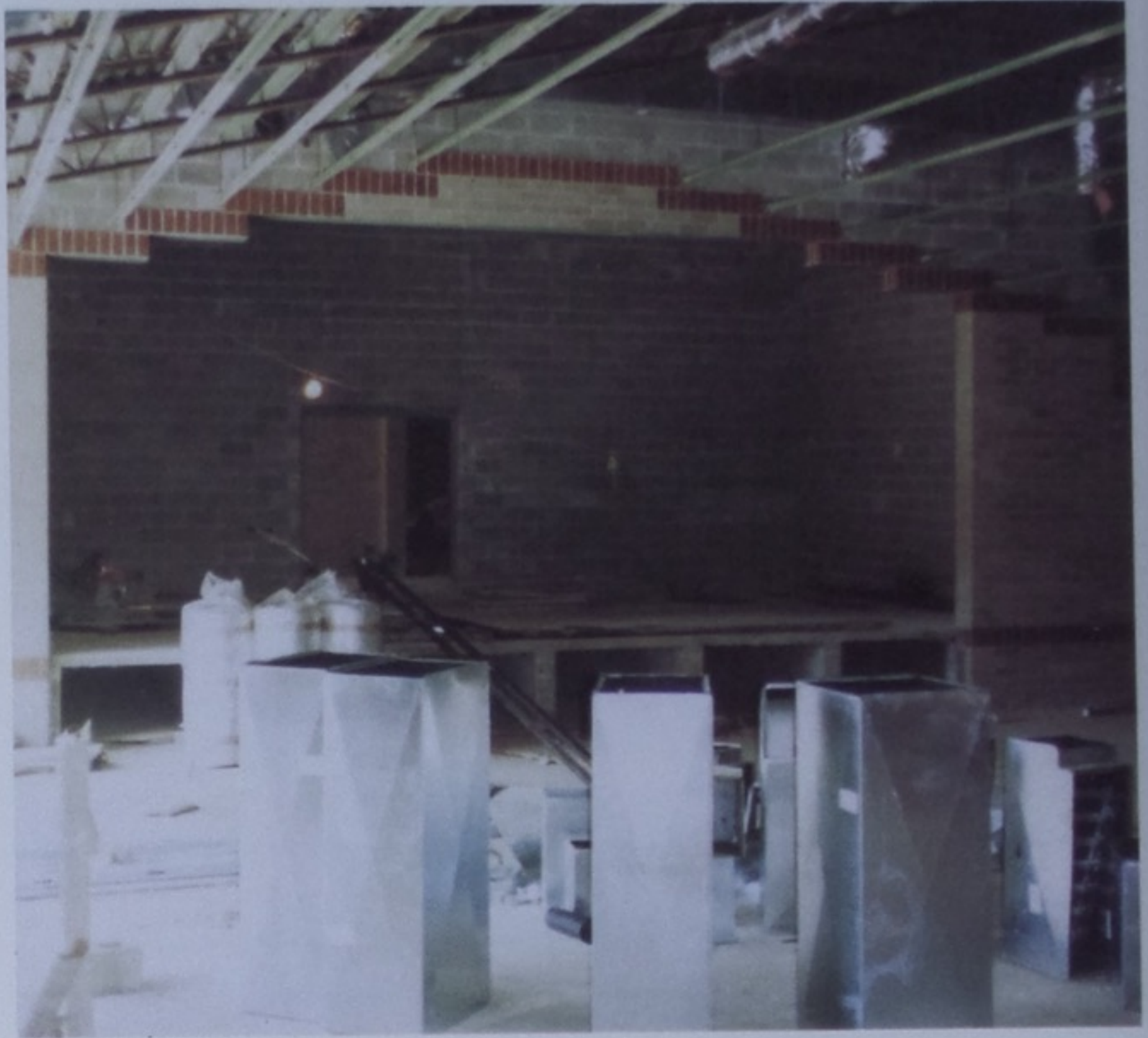
July, 1992. The construction progresses in the cafeteria area of the new high school which includes a small stage suitable for various activities and performances.
