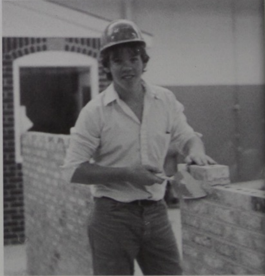
Jon Chadwick studying masonry at SCJVS, adds another brick to the wall. Jon also played first string soccer this past year.
