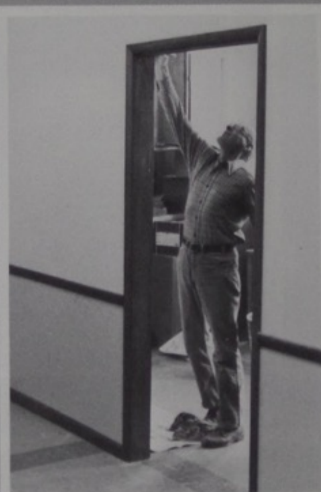
Supervisor of Maintenance, Ed Kelly paints the wall of new computer lab.
